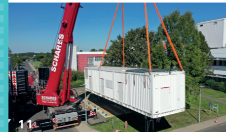
Wachtberg, September 7 Loading and assembly of the new GESTRA container on the institute's premises
